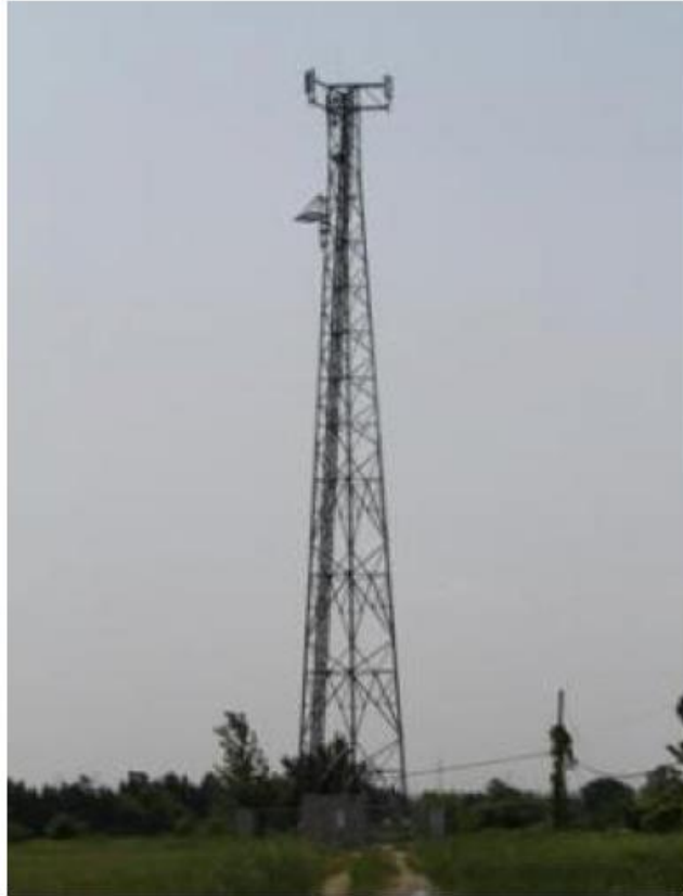
Figure 2- Example of Self Support Tower (Type S)
