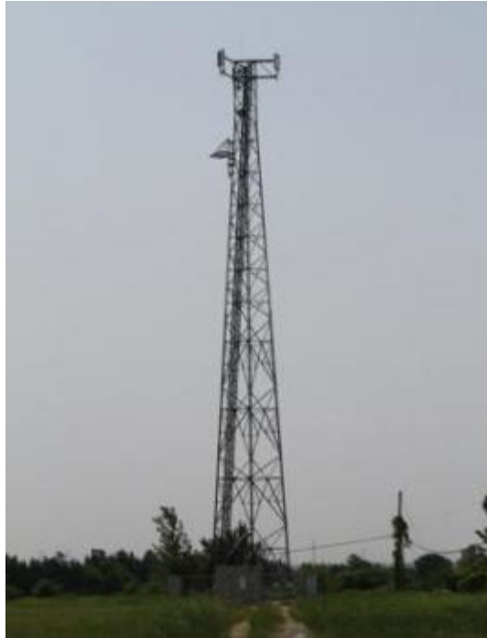
Figure 2- Example of Self Support Tower (Type S)
